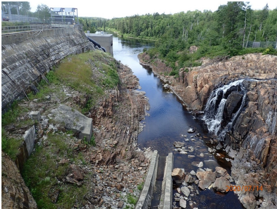
Figure 2-6 Stinson Spillway: Leakage Flow Only
