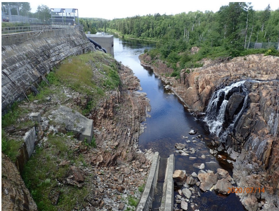
Figure 2-6 Stinson Spillway: Leakage Flow Only
