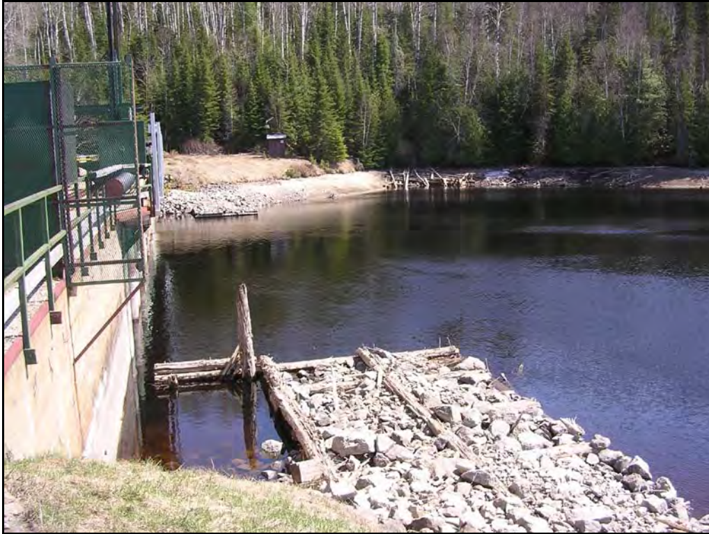
Upstream side of Mattagami Lake Dam showing old rock filled crib structures.
