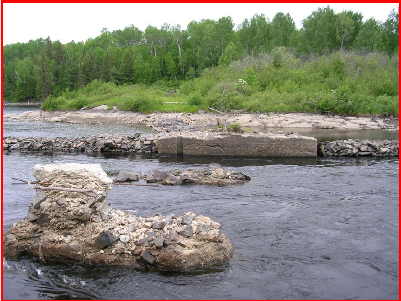
Photograph 4-2: Existing Submerged Structure at Low Water Levels in Hound Chute Generating Station Forebay Inlet
