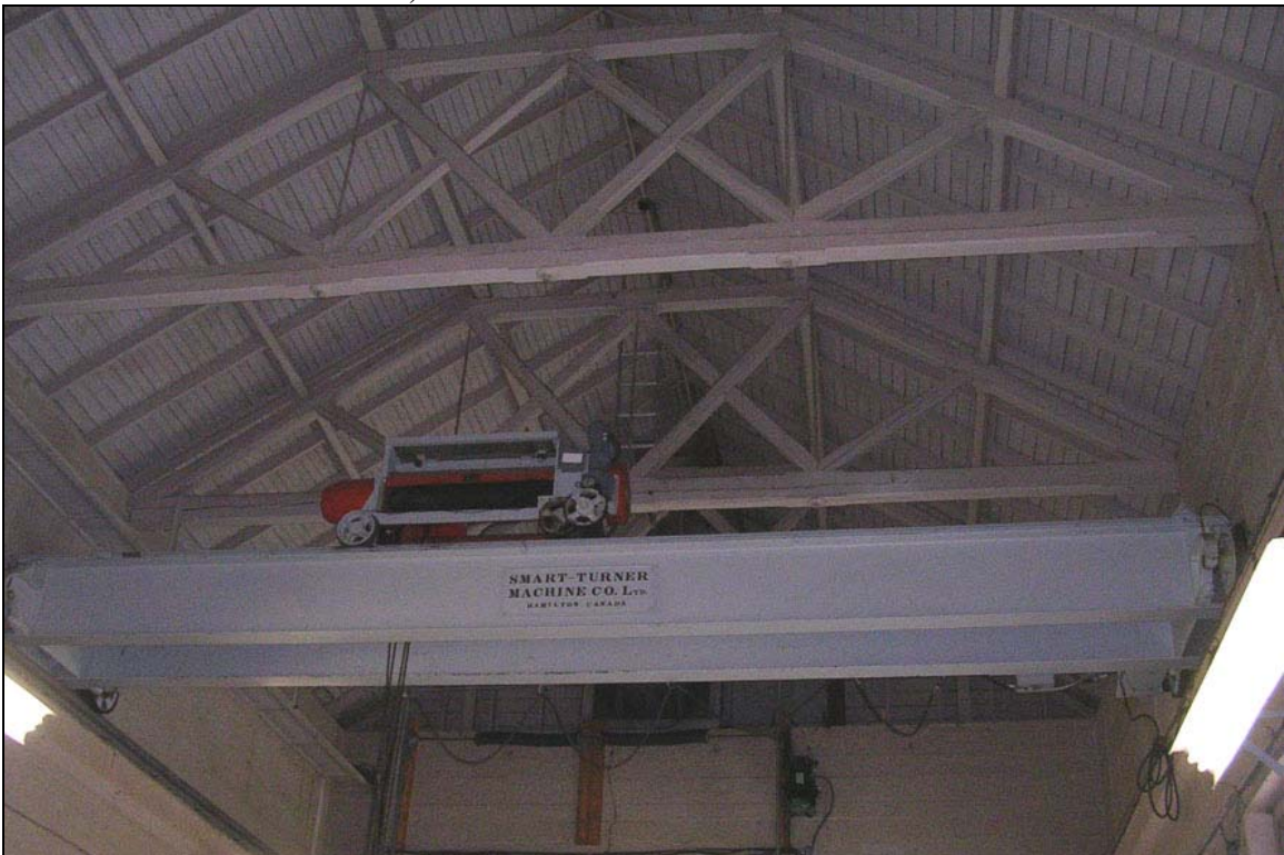
The Smart-Turner Machine Co., Hamilton manufactured the crane. Note the timber roof trusses.
