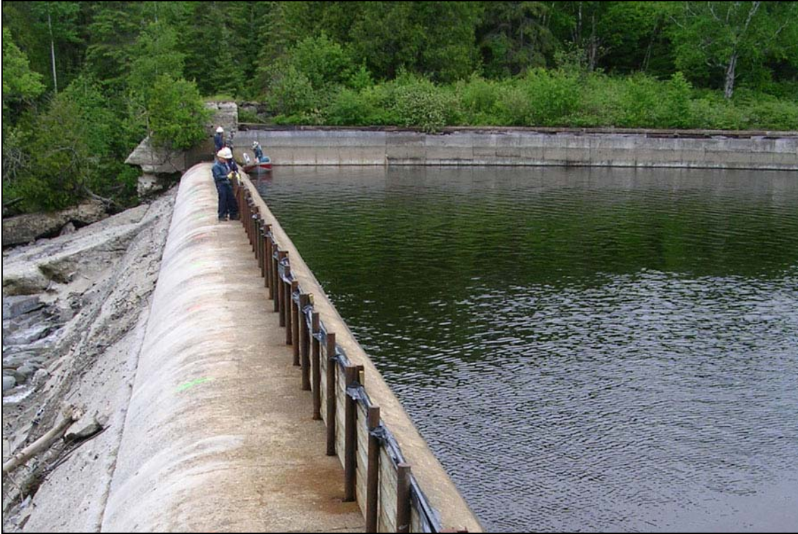
View north across the concrete dam with flashboards that replace the original timber dam.
