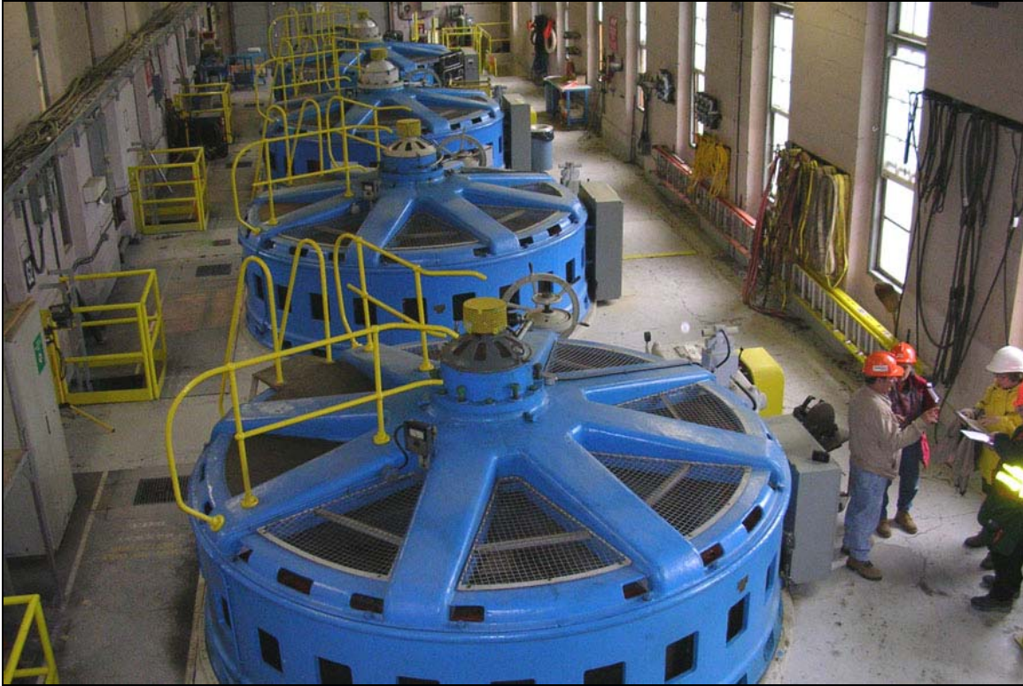
View through the interior of the powerhouse with Unit 4 in the foreground.
