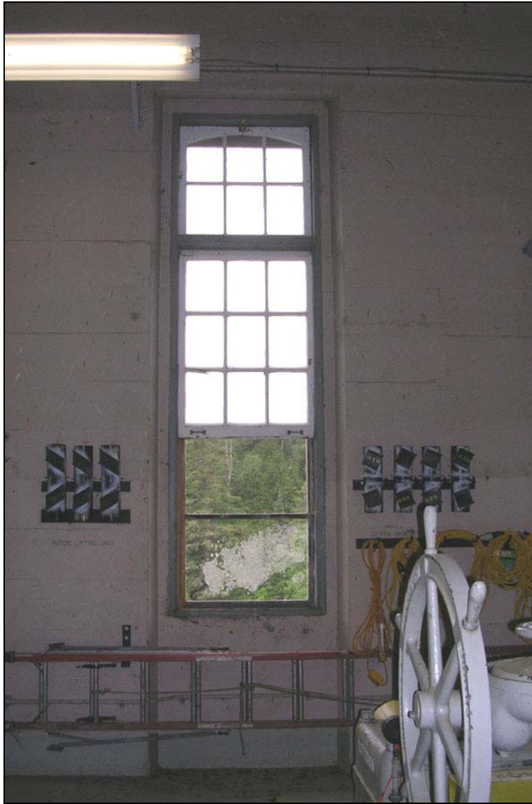
View west (downstream) of the large window on the generator floor of the powerhouse. The rectangular opening is fitted with two operable sash of nine panes of glass each with an upper transom light of six panes. Note the upper part of the transom is curved. The concrete walls were poured in horizontal sections.
