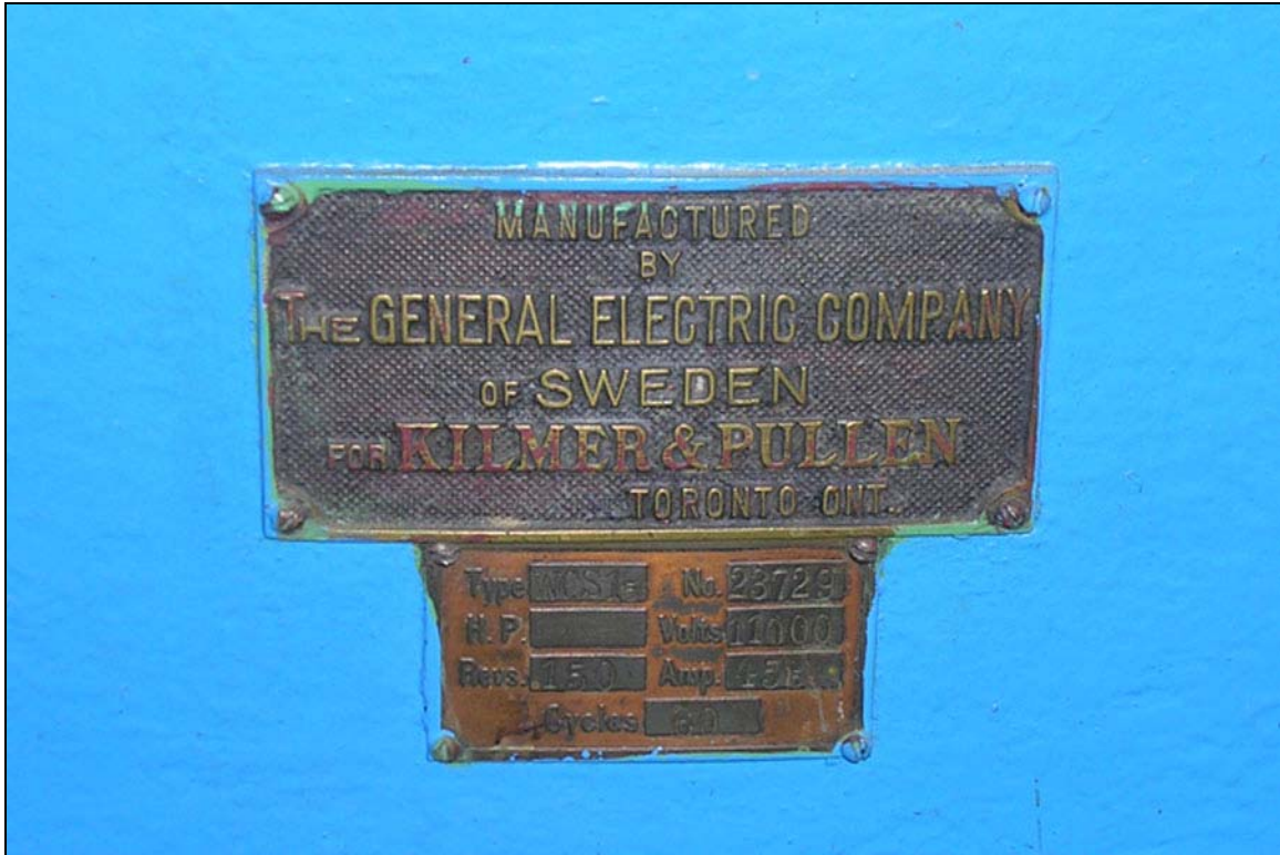
Nameplate on Unit 3 generator.
