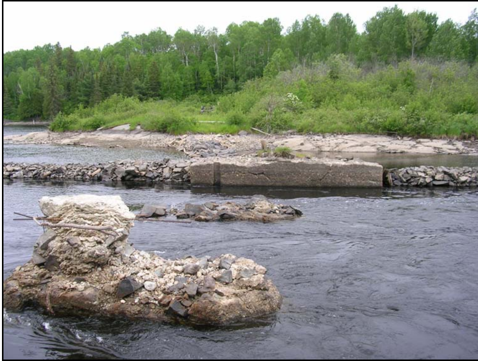
Photograph 3: Remains of old rock-filled crib and concrete bridge at upstream end of the intake channel, 2006 (Figure 2).
