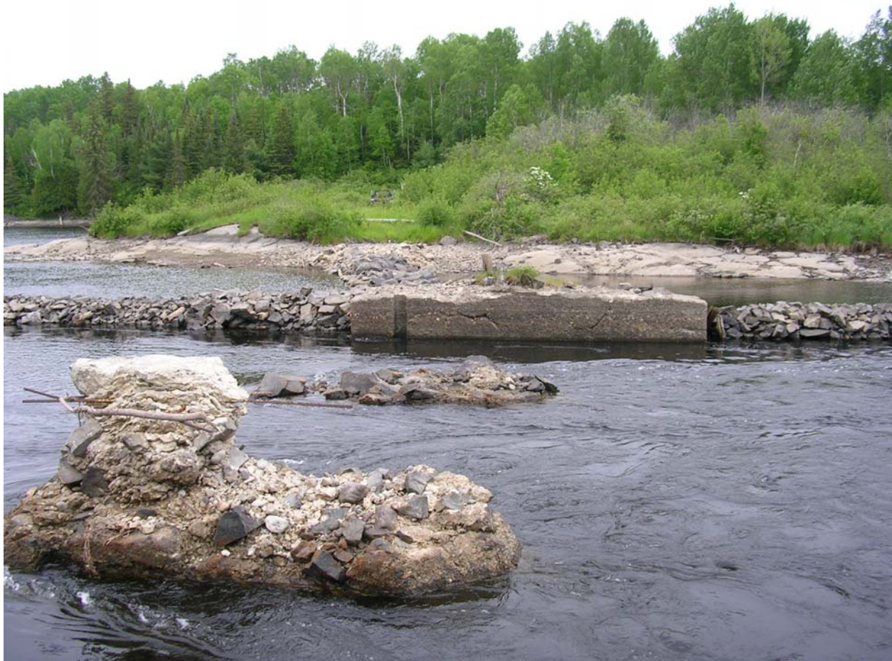
Photograph 1.2: Existing Submerged Structure at Low Water Levels, Hound Chute GS Forebay Inlet
