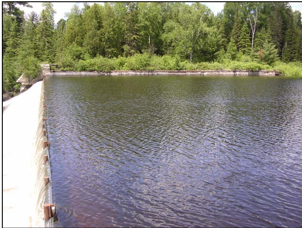
Photograph 4: View of upstream side of the crest weir at the upstream end of the spill channel. June 20, 2006.
