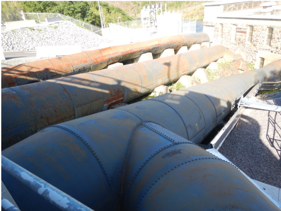
Figure 13: Penstocks showing coupling of two penstocks for Unit 3 in foreground. Note Unit 1 penstock in collapsed state.
