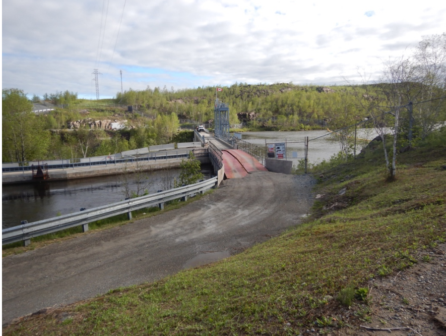
Figure 6: Access road crossing the dam and entrance to forebay canal. Note metal vehicle ramps.
