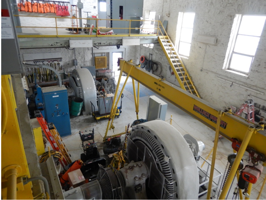
Figure 30: View from mezzanine. Unit G1 to left, Unit G2 to right. Stairs to mezzanine along south wall.
