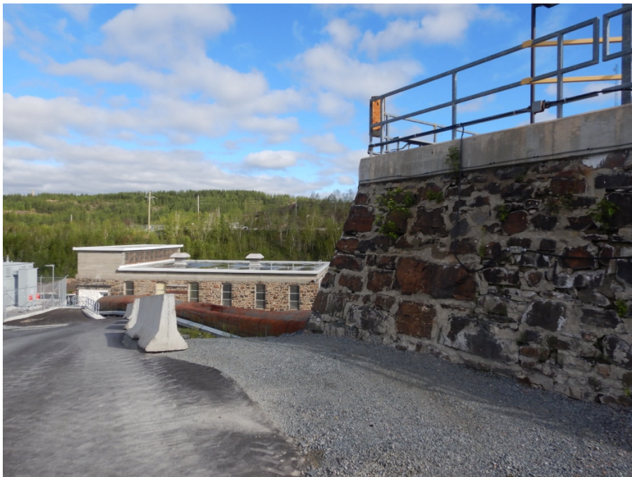
Figure 9: Downstream end of forebay canal at headworks. Note stone construction, powerhouse with flat 1954 roof in distance.
