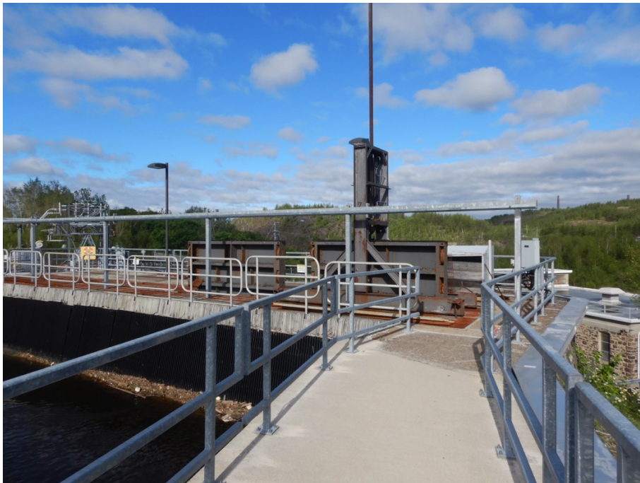
Figure 11: View of the headworks. Hoists are open to allow flow to penstock serving Unit 3.
