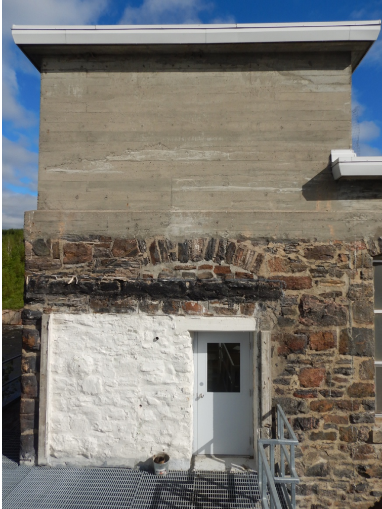
Figure 21: South wall, west end. Repurposed window to entry door, window arch above horizontal tar line marking former shed roof, and whitewashed wall section.
