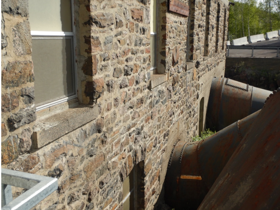
Figure 20: Entry of Unit 2 penstock, with concrete patching, and Unit 3 penstock through concrete foundation wall of the 1915 extension. Note windows in lower level.
