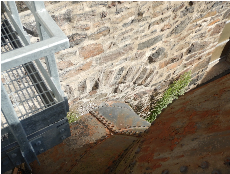
Figure 19: View of penstock to Unit 1, entry to powerhouse through stone arch. Note voussoirs and stone infill.
