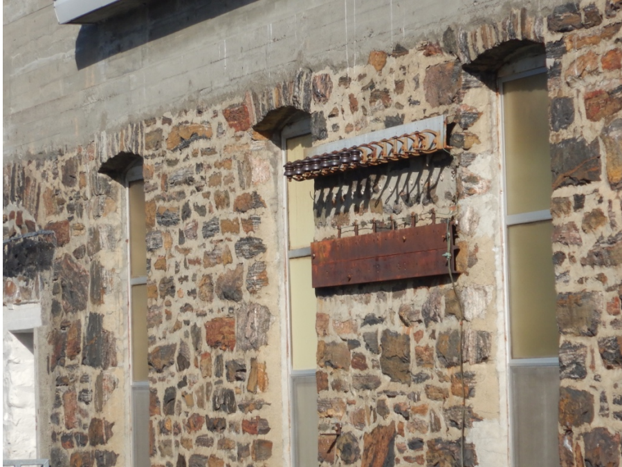
Figure 22: South wall showing wiring bracket. Note 1950s concrete wall beginning directly above the original window arches.
