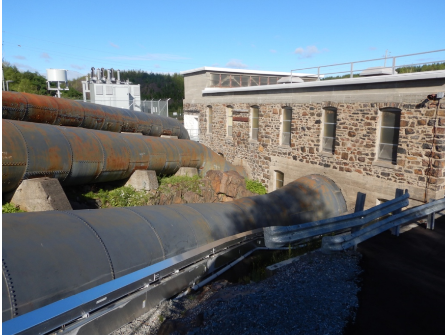
Figure 12: Penstocks as they enter the powerhouse. Unit 3 penstock, foreground, enters through concrete foundation wall. Note concrete saddles under Unit 2 penstock, and different entry angles.
