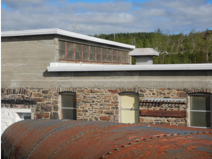
Figure 28: View across penstocks showing powerhouse roof, with lift and lights on east face.
