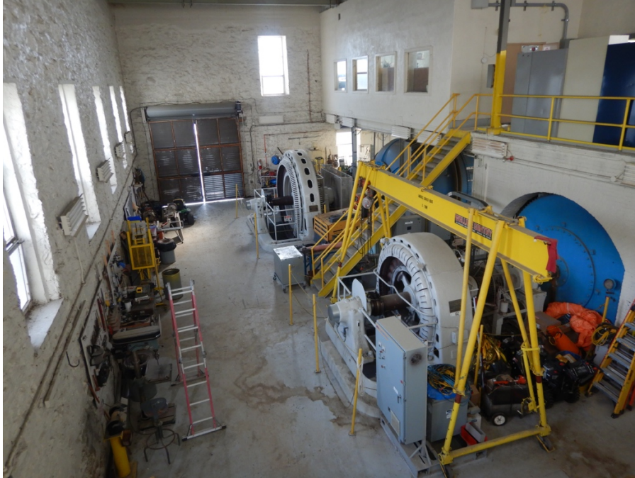
Figure 32: View from top of west stairs showing Units G2 and G3 as well as upper mezzanine.
