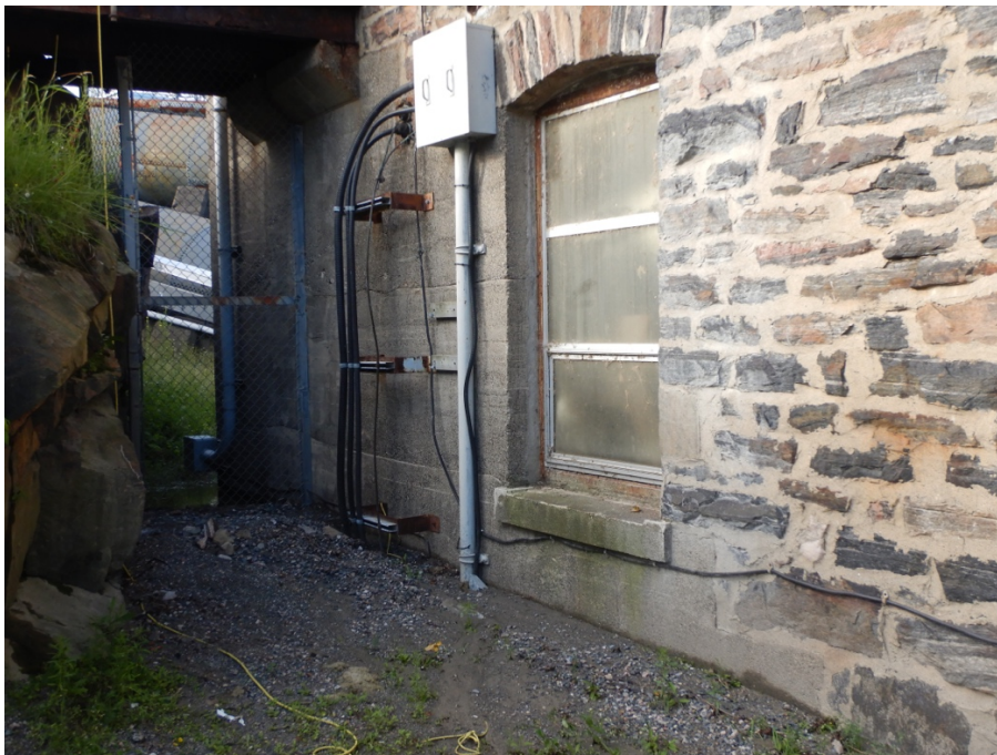
Figure 17: East wall transition from stonework to concrete foundation level. Penstocks can be seen through the chain fence.
