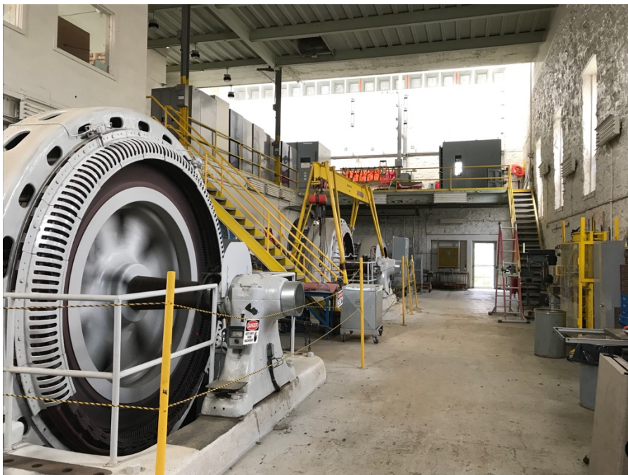
Figure 29: Powerhouse interior 2020. Unit G1 foreground, Unit G2 beneath yellow crane, and Unit G3 at end, next to service door (open) in distance.
