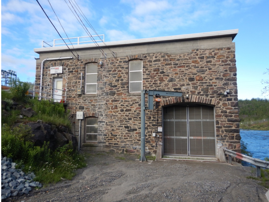
Figure 16: View of east wall, powerhouse. Window in Figure 17 on lower level to the left of the loading door.
