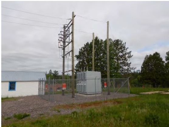
Figure 13: View west of the switchyard. The storage building is seen to the left of photo.
