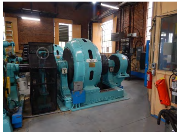
Figure 10: Bingham Chute GS, Unit 6G2 generator, with Unit 6G1 in background.
