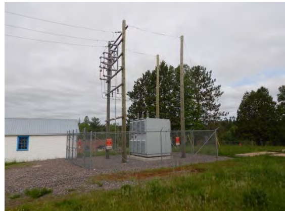
Figure 11: Bingham Chute GS, switchyard.
