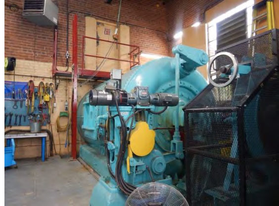
Figure 9: Bingham Chute GS, powerhouse interior, Unit 6G1 turbine and actuator.
