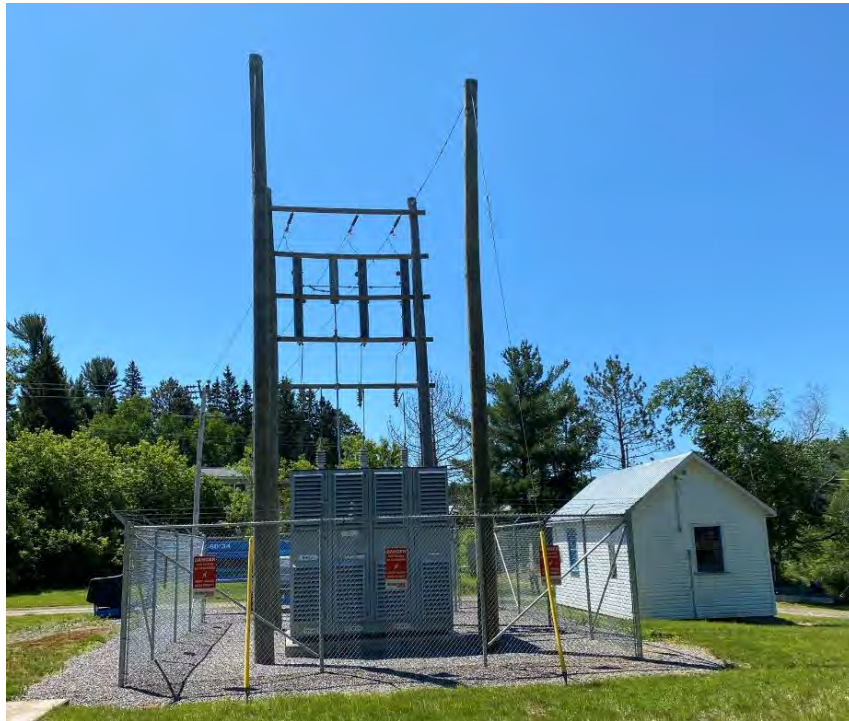
Figure 2-10 Switchyard, Transformer and Storage Shed
