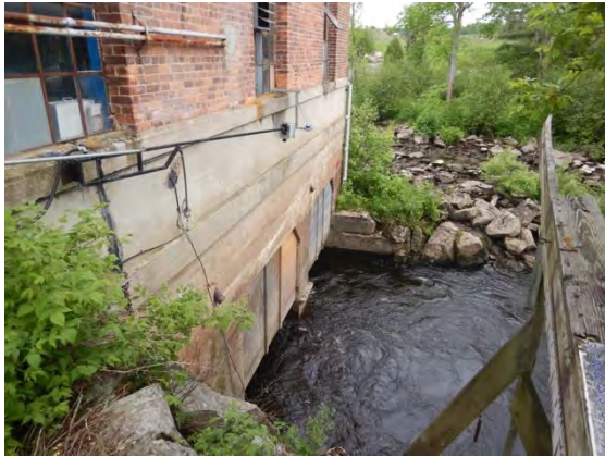
Figure 7: Bingham Chute GS, view of powerhouse, north wall with tailrace. Wood panels in openings.
