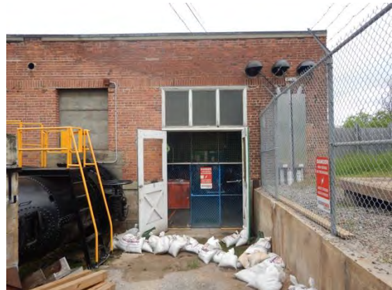
Figure 9: View north of south wall of powerhouse. Door and transom windows to be replaced.
