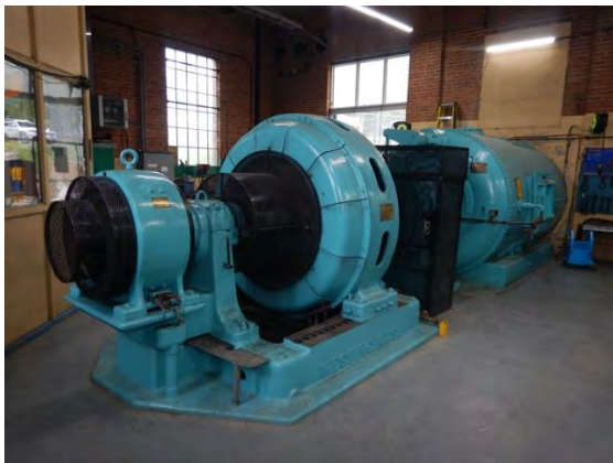
Figure 12: View east, interior, showing Unit 2. Three brass manufacturer's plates are visible in the image.
