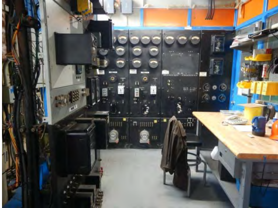
Figure 11: Electrical controls to be preserved off-site are original to the 1923 construction.
