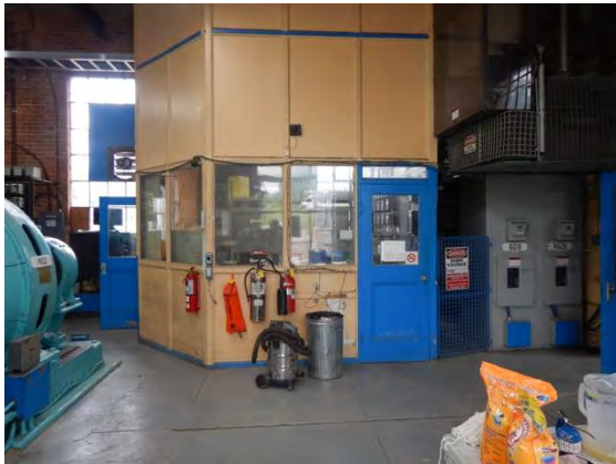
Figure 8: Bingham Chute GS, powerhouse interior showing partition and transformers.
