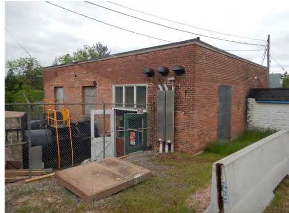
Figure 8: View northwest of brick powerhouse. Differential weathering of the brick preserves a shadow outline of the earlier addition on south wall.
